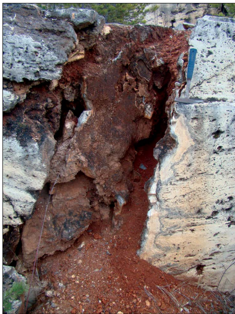
Fig. 6. Loose terra rossa infill inside the fissure within travertine visible in the quarry wall.
